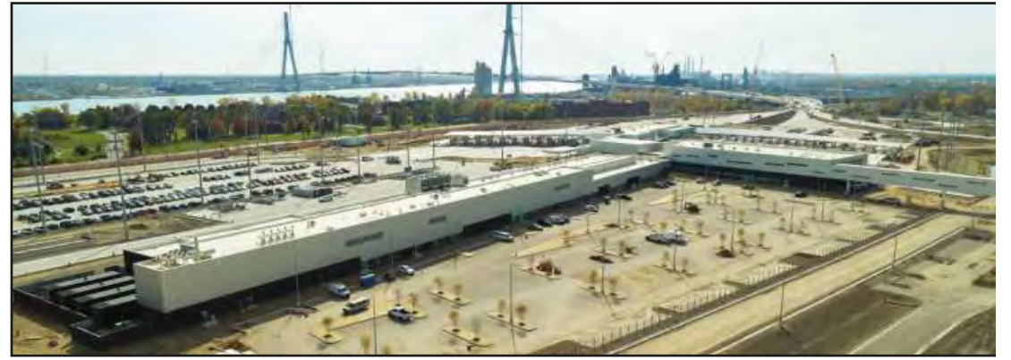
THE NEW U.S. POINT OF ENTRY behind the Gordie Howe Bridge is being erected on 167 acres in Southwest Detroit, and will include 13 structures.
