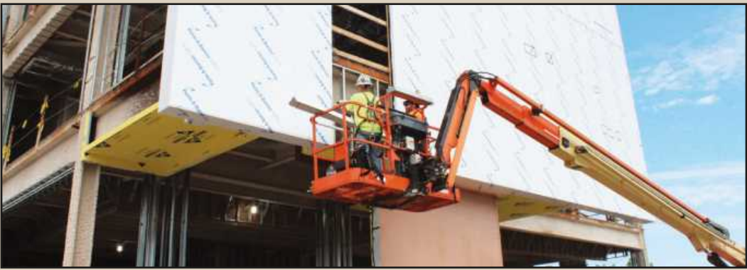
INSTALLING METAL SIDING on the OCC Culinary Institute project are Mike Hart and Eric Jesse of Sheet Metal Workers Local 80. They're employed by Liberty Sheetmetal.
