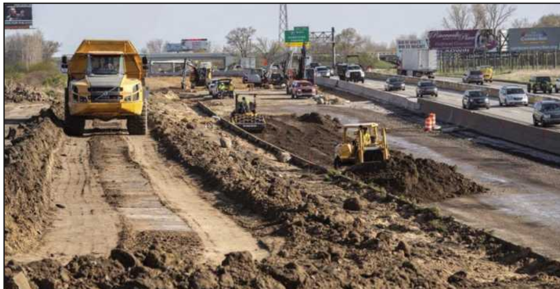
REBUILDING AND IMPROVING Michigan's 395 miles of I-75 over the years has brought a significant amount of employment to the state's road builders. Here is the I-75/M-46 rebuild project in Saginaw County, in 2021. Construction of the freeway system in Michigan and the nation was the brainchild of the Dwight Eisenhower Administration. According to the Federal Highway Administration, in June 1956, President Eisenhower signed the Federal Aid Highway Act of 1956 into law. "Under the act, the federal government would pay for 90 percent of the cost of construction of interstate highways. Each interstate highway was required to be a freeway with at least four lanes and no at-grade crossings," the FHA said.
