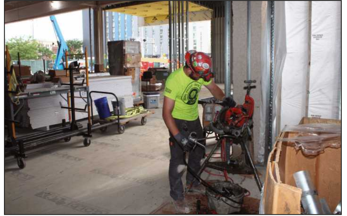
THREADING PIPE at the Oakland Community College culinary addition in Royal Oak is Drake Comeau of Sprinkler Fitters Local 704. He's employed by Shambaugh and Sons.
