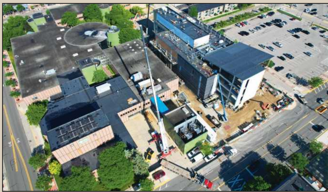
DOWNTOWN ROYAL OAK next year will be seeing a new population of students who know their way around a kitchen. Oakland Community College, in conjunction with Barton Malow and its subcontractors, is undertaking construction of a new Culinary Studies Institute addition on its existing property at Main and East Seventh Street. Photo credit: Barton Malow
