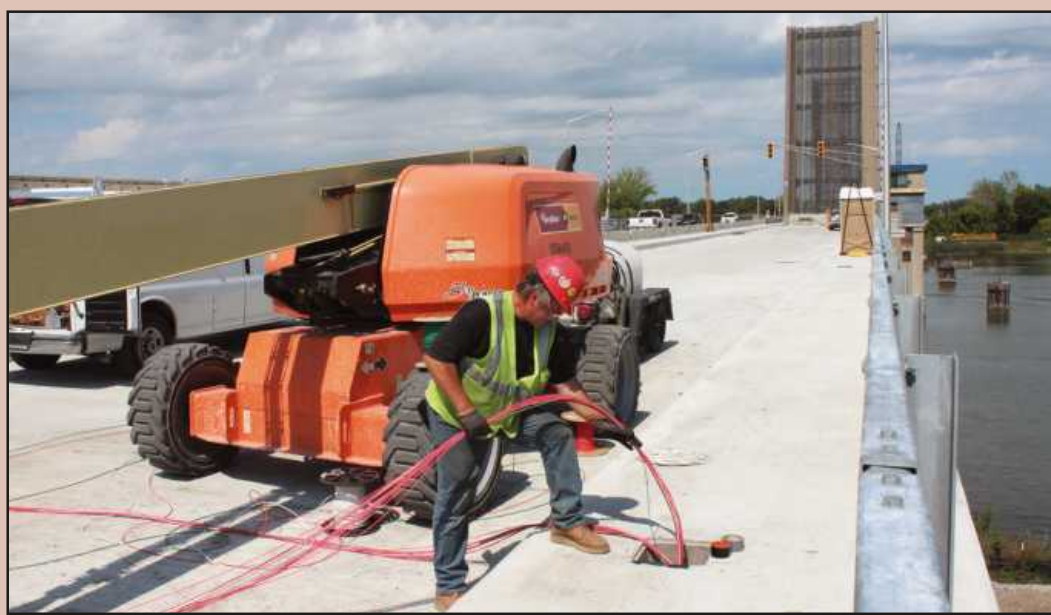
FEEDING WIRE for pump and generator controls at the Independence Bridge in Bay City is Matthew Balcer of IBEW Local 692. He's employed by Clements Electric.
