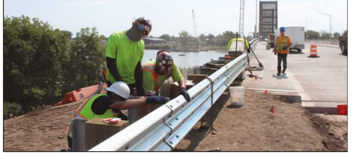
A TEAM OF IRON WORKERS Local 25 members, Jorge Willis, Kevin Palazzolo, Charles King and Eric Brecker, set guard rails on the southern approach to the Independence Bridge in Bay City. They're employed by Future Fence.
