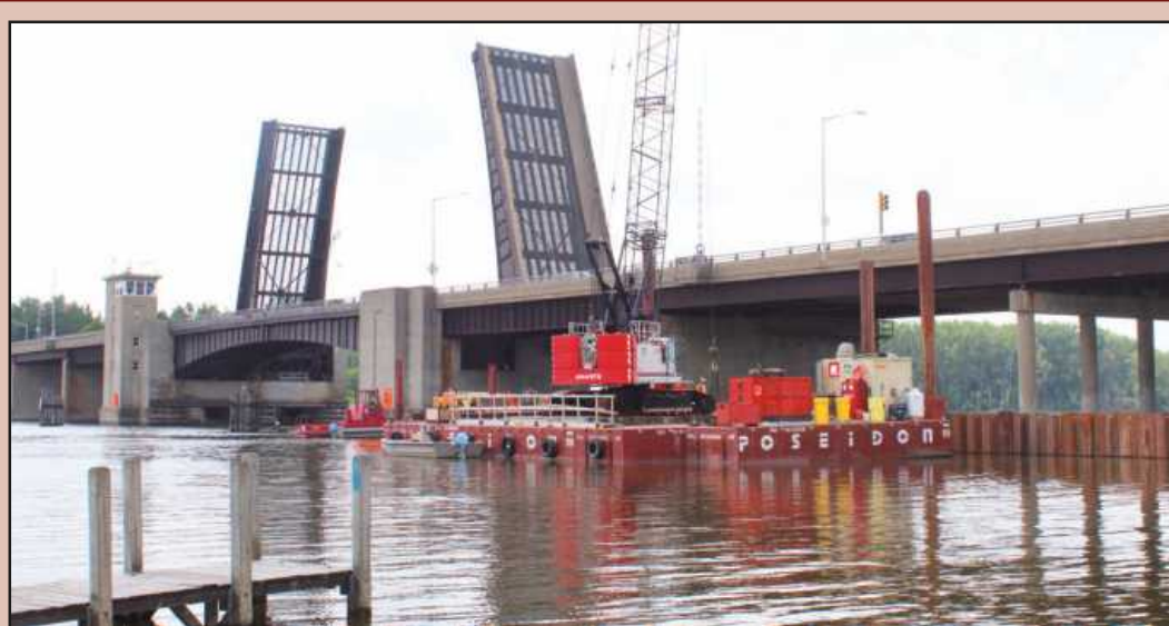
BAY CITY'S INDEPENDENCE BRIDGE, which was erected over the Saginaw River in 1973, is undergoing a complete rehabilitation project. The 1,210-foot-long bascule bridge has four independent leaves that rise and drop for ship traffic. This photo was taken in 2023.
