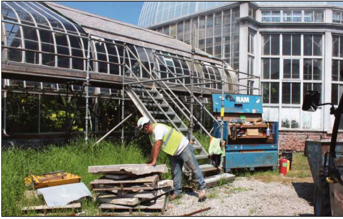
PILING OLD LIMESTONE panels which will be replaced at the Anna Whitcomb Conservatory project in Detroit is Jeremy Jewell of Bricklayers and Allied Craftworkers Local 2. He's employed by Ram Construction Services.
