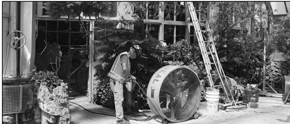
SETTING UP A WATER HOSE among plants prior to concrete cutting at the Whitcome Conservatory in Detroit is Dean Mattia of Laborers Local 1076. He's employed by Ideal Contracting.
