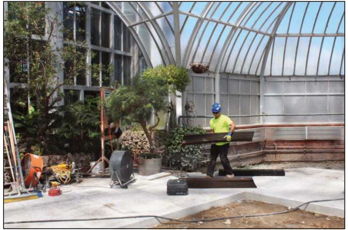
CONCRETE EXPANSION paper is hefted by Joe Peters, working for Ideal Contracting at the Anna Whitcomb Conservatory project. The Laborers Local 1076 member is working among some of the moved-aside plants in the conservatory's showroom.
