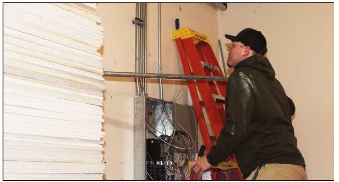
PLACING CONDUIT in a training room at the new IBEW Local 665 union hall in Lansing is journeyman Nick Blaskie of IBEW Local 665. He’s employed by H & R Electrical Contractors.
