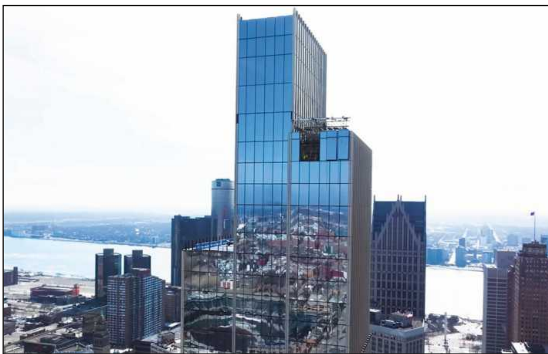
A GAP in the 47th floor of the Hudson's-Detroit tower under construction along Woodward Avenue in Detroit awaits the placement of the final section of the tower's exterior glass.
