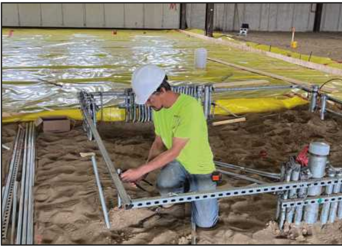
AT WORK IN THE FUTURE electric room in at the Lansing Public Safety Building is IBEW Local 665 member Matthew Ferenc. He's employed by Summit Electric.
