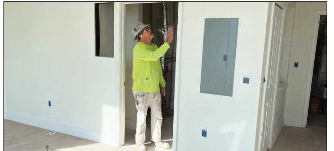
SANDING A DOORFRAME edge while painting a 14th floor apartment at the Residences @ 150 Bagley project is Roy Porter of Michigan Painters District Council Local 213. He's employed by Madias Bros.
