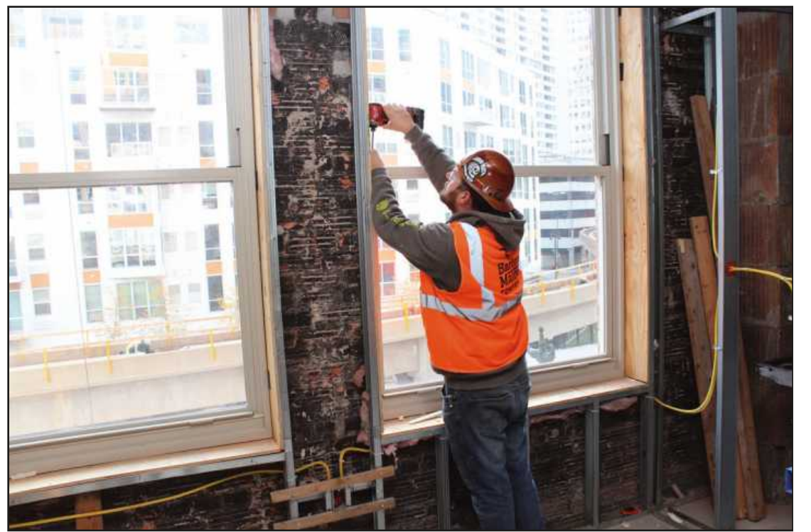
INSTALLING WINDOWS on the third floor of the Residences @ 150 Bagley project in Detroit is Curtis Braxton of Glaziers and Glassworkers Local 357. He's employed by Universal Glass. We didn't have the space to publish these photos from last year, but we do now.
