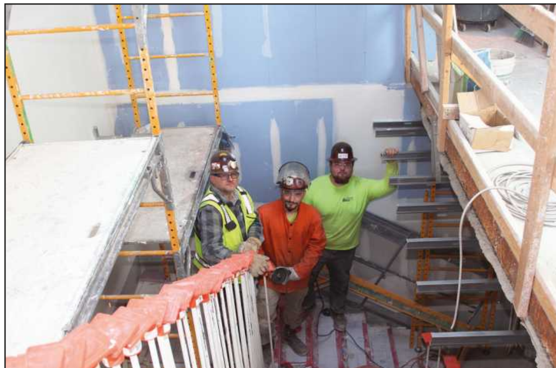
WORKING IN THE CRAMPED CONFINES of a stairwell on the 14th floor of the Book Tower project are iron workers Tim McDonald, James Viar and Aiden Viar. The Local 25 members are employed by Midwest Steel.
