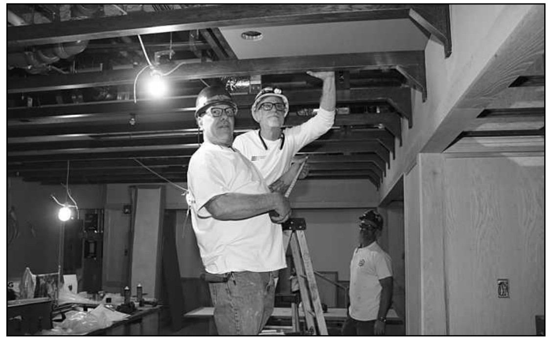
WORKING ON SETTING UP a whiskey bar in the basement of the Book Tower project in Detroit are Michigan Regional Carpenters Local 687 members Eric Schofield, Matt Rule and Eric Kramer. They're employed by Integrated Interiors.
