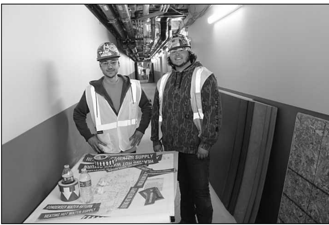
PEEL AND STICK – When pipe labels are being installed, it's a sure thing that the work is wrapping up. Applying the "Heating Hot Water Supply" and "Condenser Water Return" labels to the appropriate pipes they helped install in the basement of the Book Tower project in Detroit are Chris Xenos and Zach Kessey. The Pipe Fitters Local 636 members are employed by Complete Mechanical.
