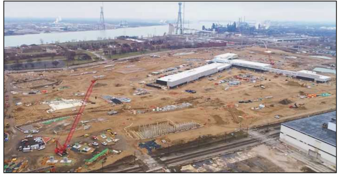
PROGRESS IS CONTINUING on the massive 167-acre Point of Entry for the Gordie Howe Bridge in Southwest Detroit. It will be one of the largest border points of entry in North America, and contain inbound and outbound inspection facilities, control booths and other facilities.
