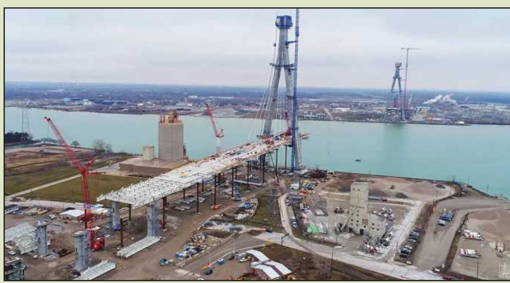
AT THE GORDIE HOWE BRIDGE site, the trades have about 100 feet to go before the concrete tower pylon is complete at 722 feet.
