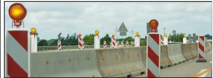
ROAD BARRIERS increase worker safety.
