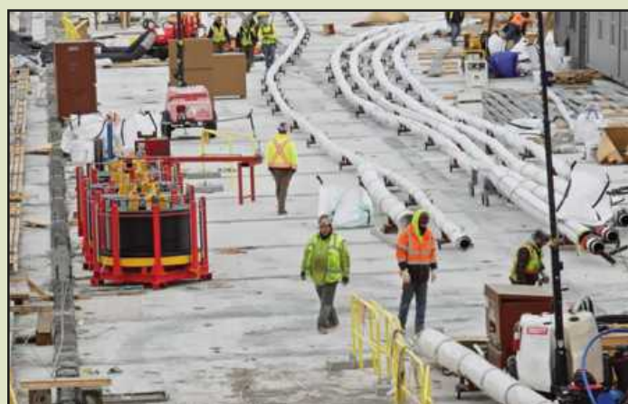
THE BUSY DECK of the Gordie Howe Bridge, on the Detroit side.
