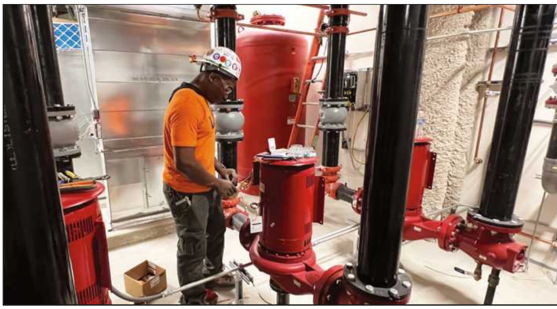
WIRING A PUMP MOTOR in the mechanical penthouse of the new Oakland Community College culinary school in Royal Oak is electrician Davian Johnson. The IBEW Local 58 member is employed by Centerline Electric.
