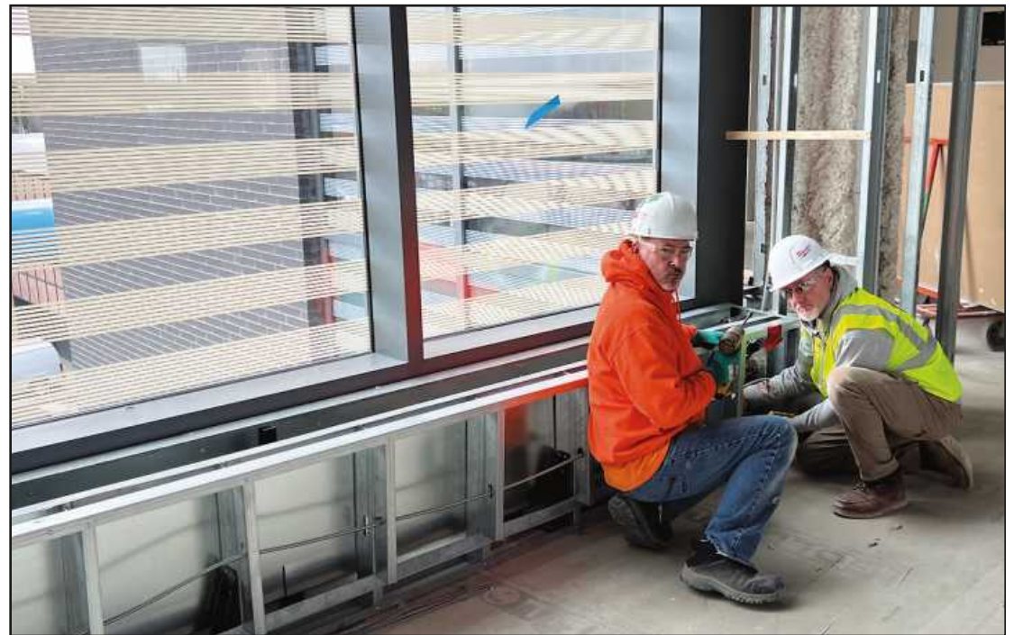
SETTING A HEAT SHIELD for a third floor fin tube radiator at the Oakland Community College Culinary School in Royal Oak are (l-r) sheet metal workers Craig Murdock (Local 80) and Bill Brooks (Local 7). They're employed by S & G Sheet Metal.
