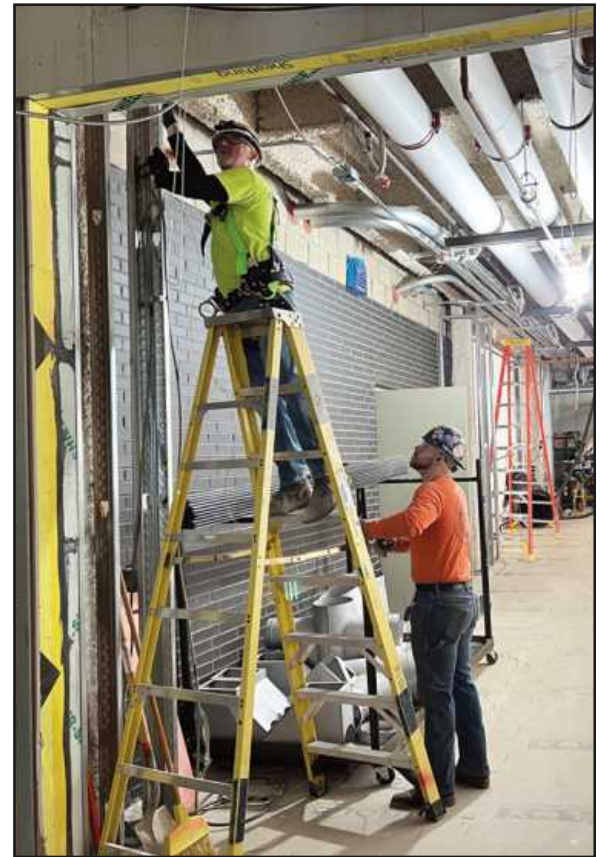
SETTING HVAC controls at the Oakland Community College Culinary School in Royal Oak are electricians Charles Cole (on the ladder) and Justin Savine. The IBEW Local 58 members are employed by Compass Technologies.
