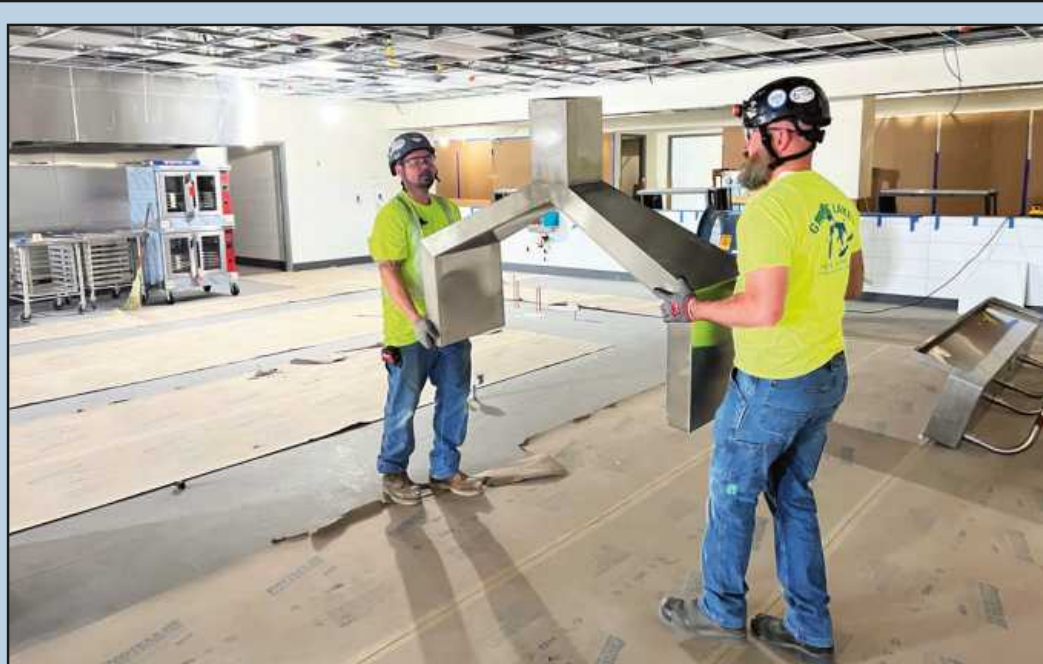
A “PANT LEG” exhaust fixture that will be placed above a dishwasher in a third-floor kitchen at the culinary school under construction at Oakland Community College in Royal Oak is on the move, hauled by Scott Doyle and Ken Palmeri. The Sheet Metal Workers Local 80 members are employed by Great Lakes Hotel Supply.
