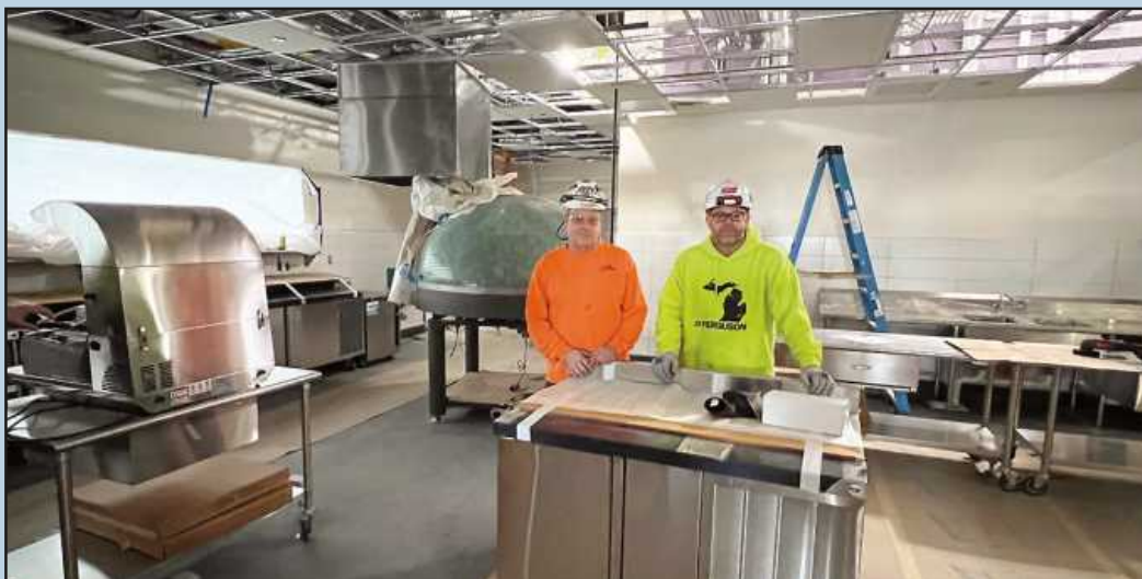
SURROUNDED BY STAINLESS STEEL, plumbers Tim Music and Joe Darmafill looked up from what they were doing to have their photo taken in a third-floor kitchen at OCC's culinary school. The Plumbers Local 98 members are employed by Western Mechanical. Truly a full-service kitchen: the green half-orb behind them is a pizza oven.
