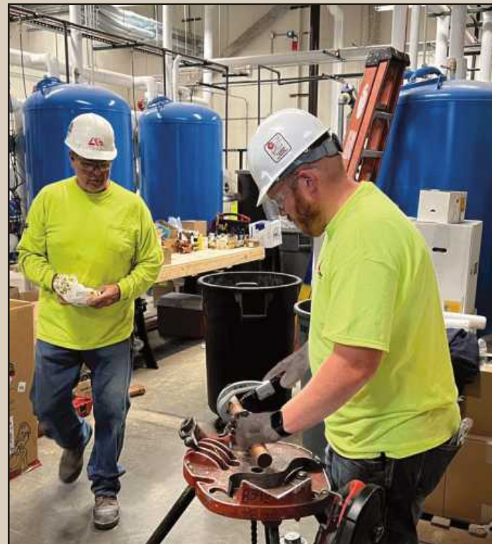
CUTTING 1.5-INCH copper pipe in the utility plant at the Firekeepers project are (l-r) Ron Morsaw (Plumbers and Pipe Fitters Local 174) and James Blair (Plumbers and Pipe Fitters Local 333). They're employed by Andy J. Egan.
