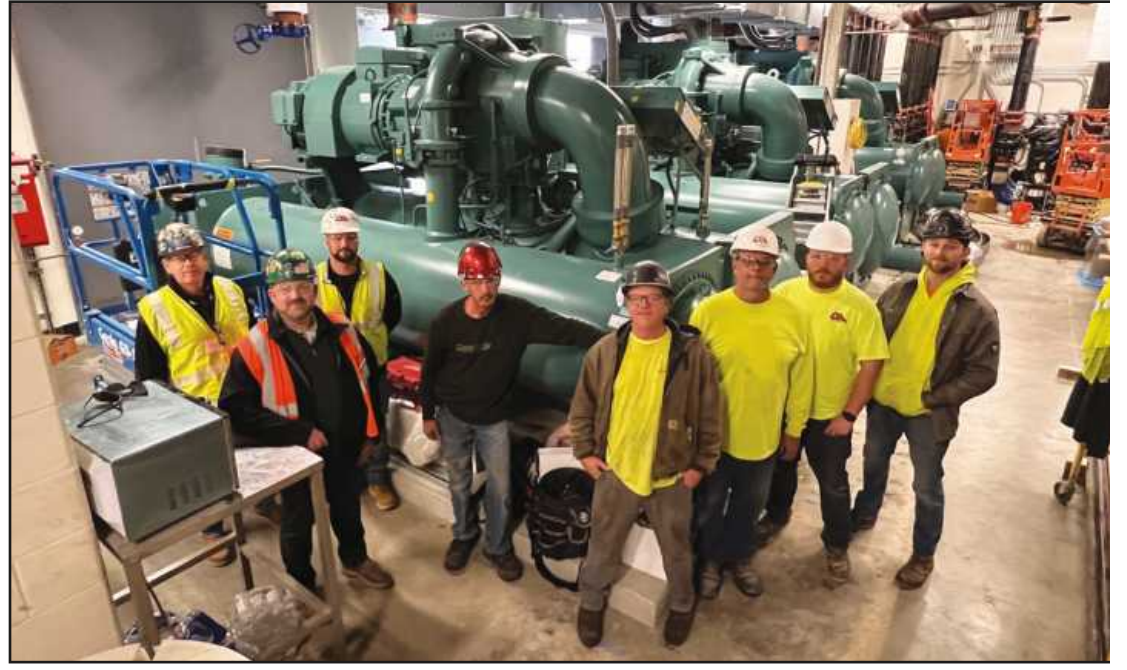
A GROUP OF CHILLERS provide the backdrop at Firekeepers Casino Hotel for this group of pipe trades workers, who we asked to assemble for a photo. They include (l-r) Plumbers and Pipe Fitters Local 333 BA Joe Michilizzi, Local 333 BA Nick Asher, Andy J. Egan Design-Build Project Manager Joe Williams (UA Local 174), Joel Kinney (Local 333), Todd Stuke (Local 333), Ron Morsaw (Local 174), James Blair (Local 333), and Ryan Vought (Local 333).
