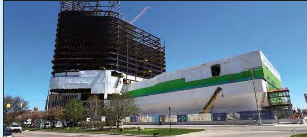
THE WEST GRAND BOULEVARD face of Henry Ford Health's Destination Grand, was still partially under its winter wraps in mid-April. Skywalks will connect the facility with Henry Ford Hospital across the street and the health care facility's cancer center next door. The Building Tradesman has yet to be granted access to take photos inside the project.
