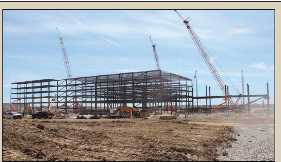
WHAT WILL BE THE largest building on the grounds of the former Silverdome, a five-story 3.5 million square-foot warehouse/fulfillment center, goes up on the new Amazon-Pontiac site.
