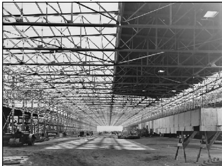
THE WILLOW RUN plant under construction in 1941. Completed with about seven million square feet, some production began at the plant in September 1941.
