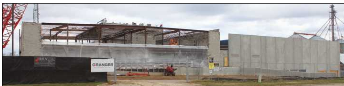
INGHAM COUNTY'S new Justice Complex, now being built by Granger Construction and its subcontractors, will encompass 169,472 square feet, and replace an outmoded facility that dates to 1964.
