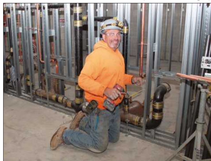
ROUGHING IN plumbing at the Ingham County Justice Complex is Brian Koffong of Plumbers and Pipe Fitters Local 333. He's employed by John E. Green.
