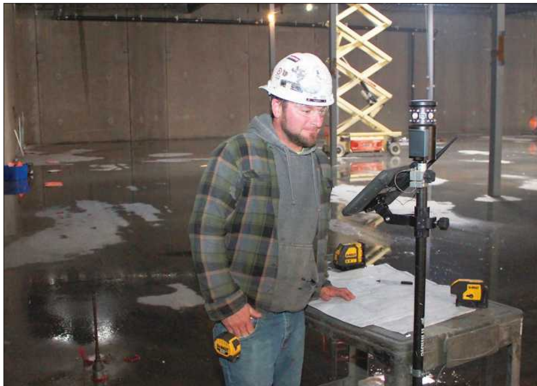
GAZING AT A TRIMBLE — an electronic device which helps turn drawings into measurements and facilitates the placement of ductwork — is Travis Drennan of Sheet Metal Workers Local 7. The Applegate tinknocker is working at the Ingham County Justice Complex in Mason.
