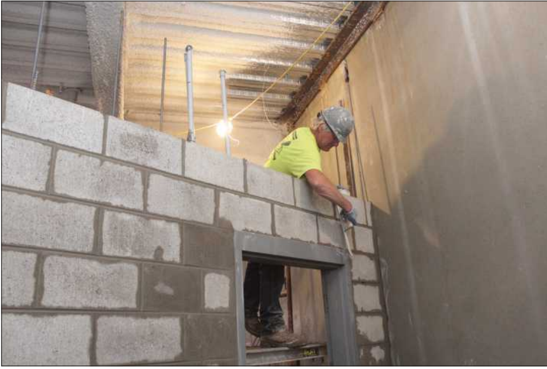
SETTING MORTAR FOR BLOCK WALLS in one of the rooms without a view at the Ingham County Justice Complex are masons Kent Buta, above, and Clifton Williams, below, of Bricklayers and Allied Craftworkers Local 2. They're employed by Davenport Masonry.
