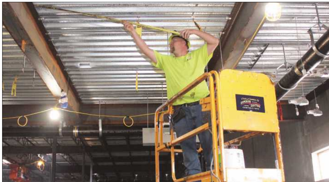
TAKING A MEASURE for conduit at the Ingham County Justice Complex is Dennis Meyers of IBEW Local 665. He's employed by Superior Electric.
