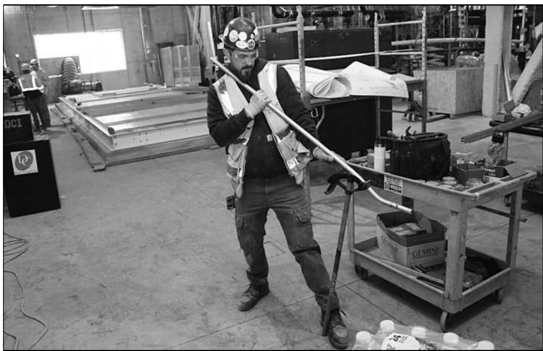
BENDING A SECTION of conduit while working at the Trinity Health-Brighton hospital project is Evan Olds of IBEW Local 58. He's employed by Centerline Electric.
