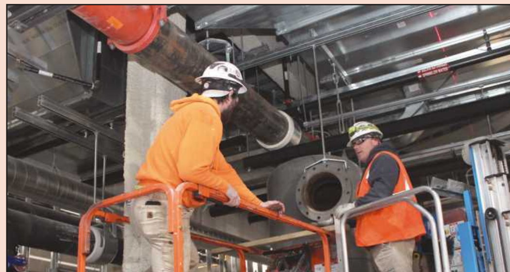
GETTING READY TO SET a 12-inch chilled water Victaulic fitting at the Trinity Health-Brighton Medical Center are pipe fitters Rhett Lowe (Plumbers and Pipe Fitters Local 333) and William Thomas (Plumbers and Pipe Fitters Local 190). They're employed by John E. Green.
