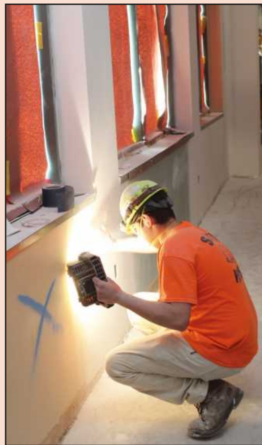
SANDING DRYWALL in the revamped portion of the existing Trinity Health-Brighton Medical Center is Braulio Galindo of Michigan Painters District Council Local 2353. He's employed by ACP.
