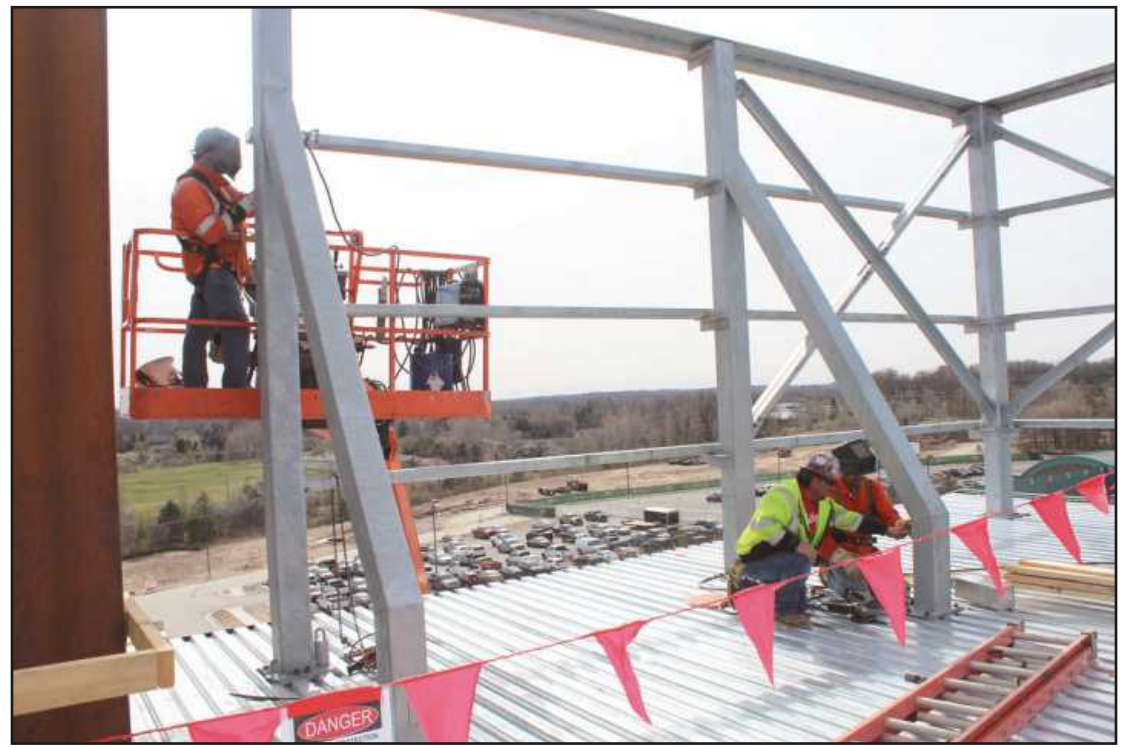
ERECTING A SCREEN WALL on the roof of the Trinity Health-Brighton hospital project are (l-r) iron workers John LeClair, Jason Wikaryasz and Scott O'Lelley. The Local 25 members are employed by Sterling Erectors.
