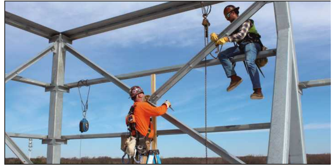
ASSEMBLING A SCREEN WALL atop the Trinity Health-Brighton hospital project are (l-r) iron workers Edward Lane and Noah Davenport. The Local 25 members are employed by Sterling Erectors.
