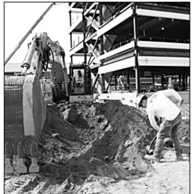
DOING SOME DIGGING at the Trinity Health-Brighton hospital project are Wyatt Suttle, with the shovel, of Laborers Local 499, and Operating Engineer Ron King of Local 324, behind the controls of a Cat 320 excavator. They're employed by Eagle Excavating.
