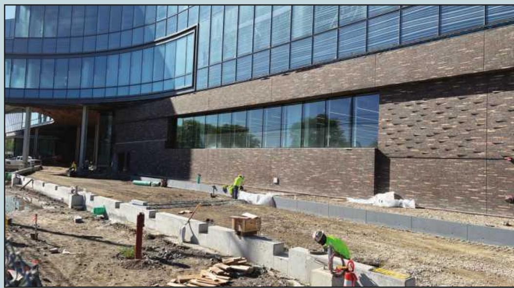
READYING THE MAIN entrance of the Ford Central Campus Building in Dearborn for concrete work are (l-r) laborers Saul Reyno (Local 1191, employed by Site Development) and Zack Parker (Local 1076, Fessler and Bowman).
