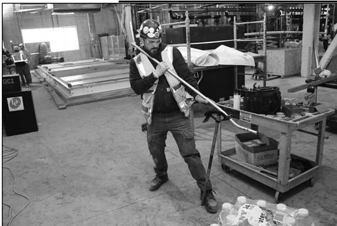
BENDING A SECTION OF CONDUIT while working at the Trinity Health-Brighton hospital project is Evan Olds of IBEW Local 58. He's employed by Centerline Electric.
