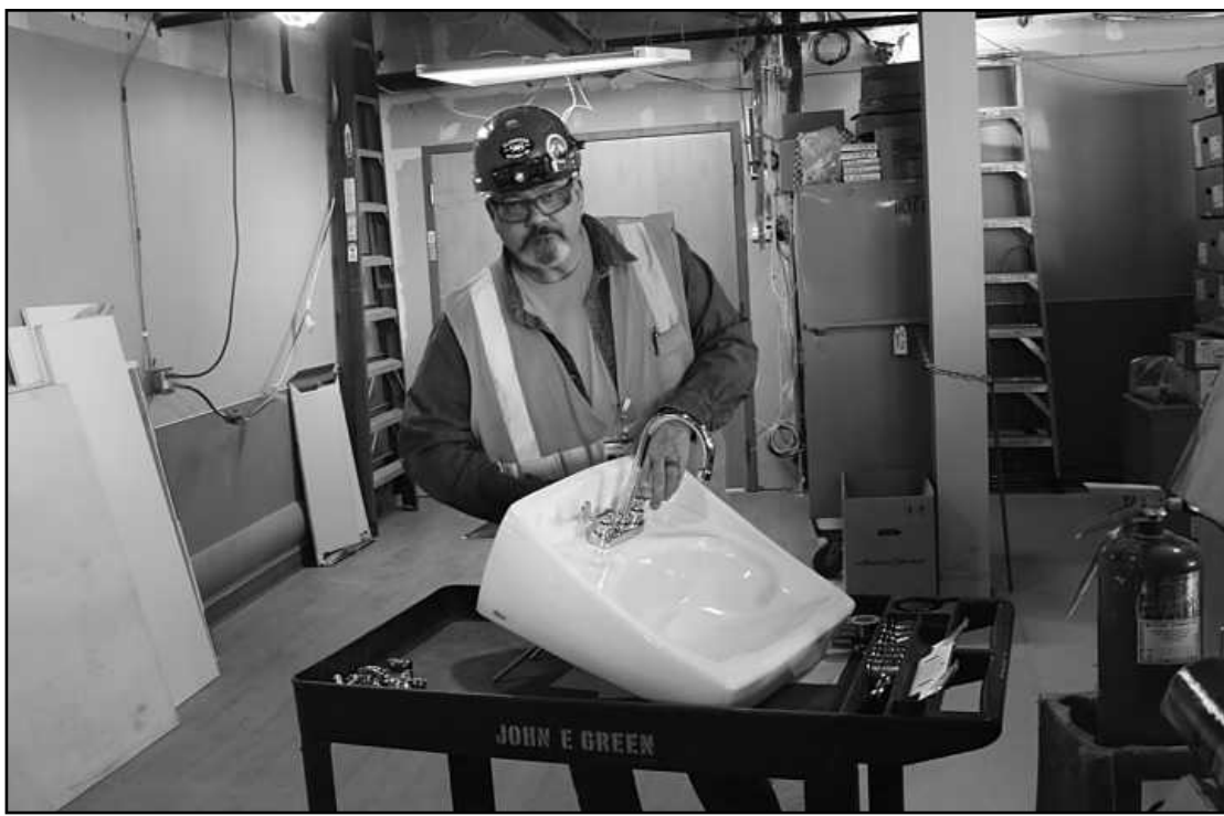
SETTING SINK HARDWARE in the existing Trinity Health-Brighton hospital is Bill James of Plumbers Local 98. He's employed by John E. Green.
