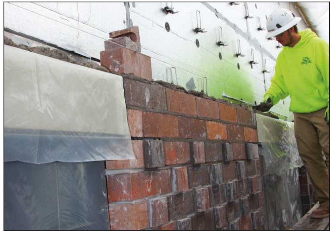
LAYING A BRICK WALL at the Hannahville Indian Community’s new Governmental Services and Health Clinic Building is Colton Lindemann of Bricklayers and Allied Craftworkers Local 2. He’s employed by Miron Construction.
