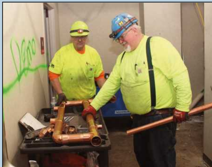
ASSEMBLING A HEADER on the seventh floor of the Genesee County building for its new heating supply and return system are plumbers David LaForest and Mike Vondra. The UA Local 370 members are employed by Platinum Mechanical.
