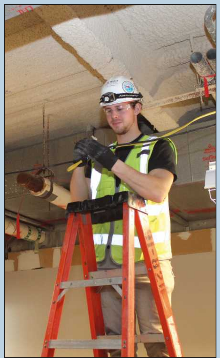
Nicely spliced SPLICING WIRING for a temporary lighting fixture on the second floor of the Genesee County Building project in Flint is Eric Hunsinger of IBEW Local 948. He's employed by Walker Electric.
