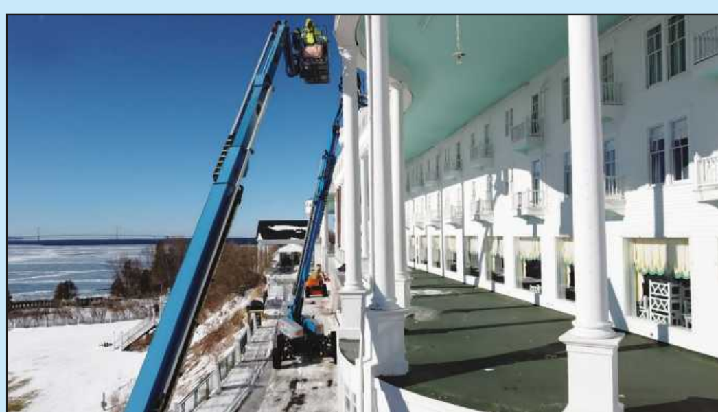
UNION CARPENTERS employed by Spence Brothers worked outside during the frigid offseason to renovate the Grand Hotel on Mackinac Island. Image credits: Spence Brothers
