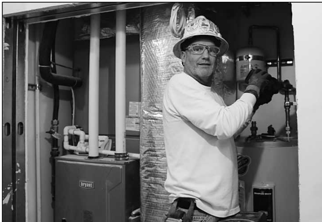
SETTING UP WATER HEATER piping in a 16th floor condominium unit at the Exchange Building in Detroit is Plumbers Local 98 member Jerry Wilson. Employed on this project by Western Mechanical, Jerry insisted that his photo caption include "proud 34-year member of Local 98." Consider it done.
