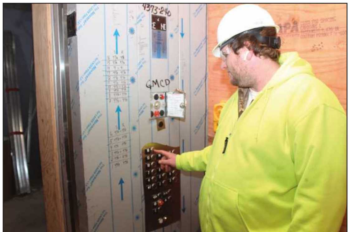
GOING UP: Operating one of the elevators at the Exchange Building project in Detroit is Michael Wallace. The Elevator Constructors Local 36 member is employed by Kone.
