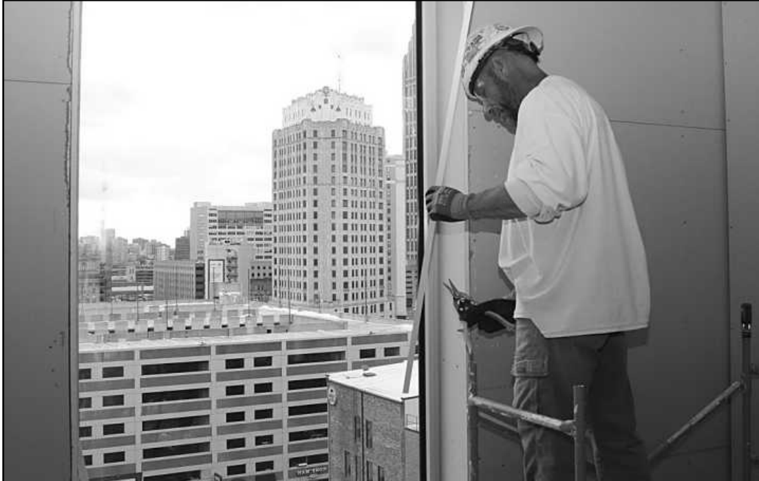
SNIPPING A SECTION of corner bead while finishing drywall in an 8th floor apartment at the Exchange Building project in Detroit is Rick Wetmore of Michigan Painters District Council 1M, Local 2353. He's employed by Barton Malow.
