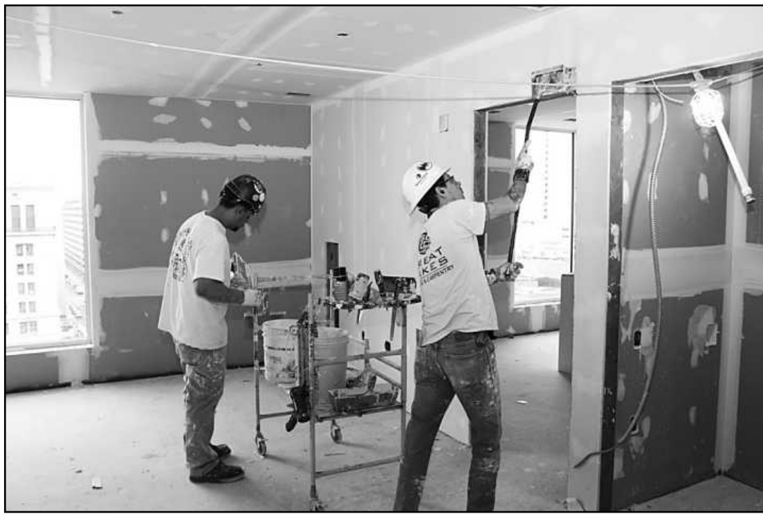
SANDING DRYWALL in a ninth floor apartment at the Exchange Building in Detroit are Ryan Crews and Roberto Sanchez of Painters District Council 1M Local 2352. They're employed by Barton Malow.
