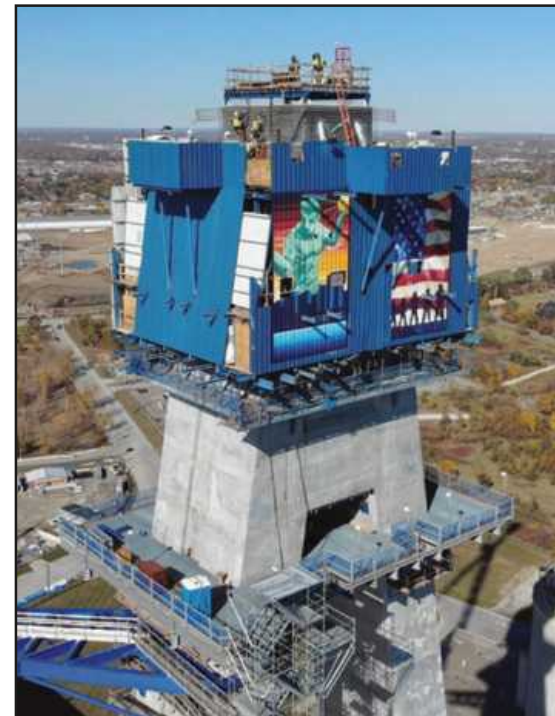
THE TOP OF THE TOWER leg on the U.S. side of the Gordie Howe Bridge, which will receive the anchor boxes, above.
