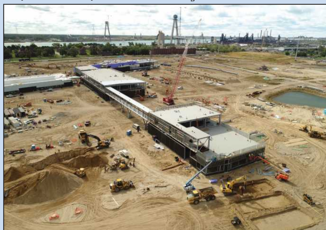
A MASSIVE 167-acre-swath of land in Southwest Detroit has been cleared, and construction is well under way on the new Detroit Point of Entry buildings. The Windsor-Detroit border crossing is the busiest in North America. The Gordie Howe bridge towers are in the background. Image credits: Bridging North America
