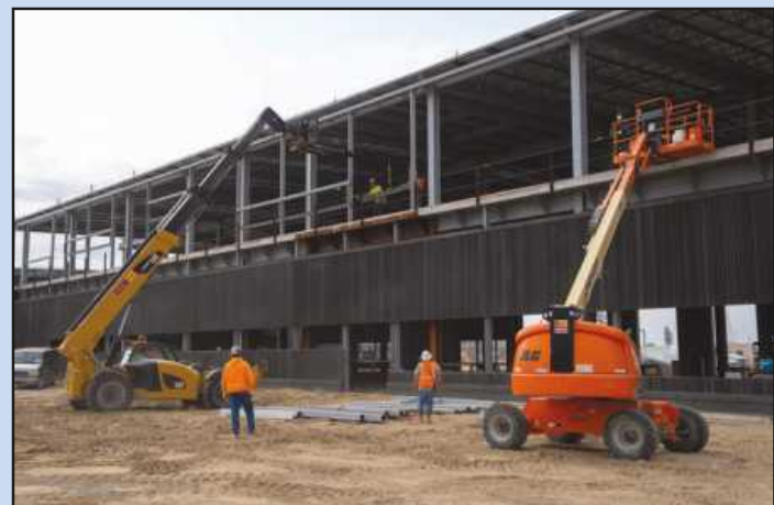
CONSTRUCTION on the U.S. Port of Entry buildings behind the Gordie Howe Bridge in Detroit.
