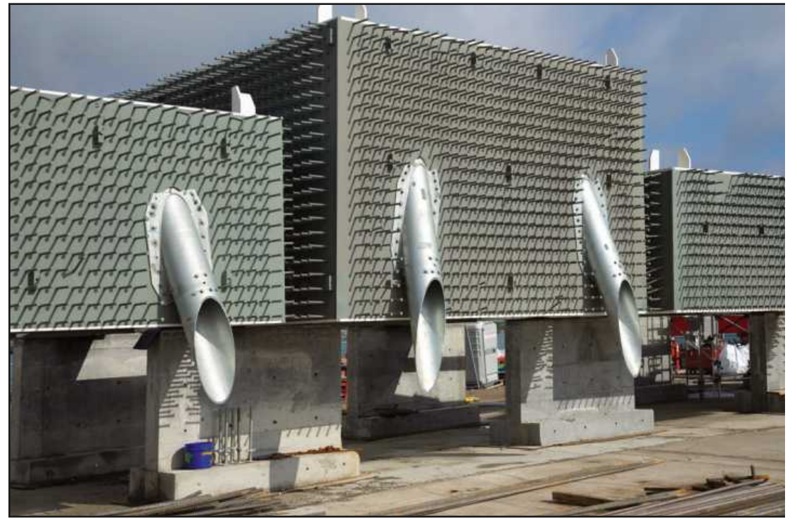
ANCHOR BOXES at the Gordie Howe Bridge site are among 35 that will be installed into the top of the Canadian and U.S. towers. These boxes will house the cables connecting the bridge deck to the towers. As of Nov. 22 five boxes have been installed in the Canadian tower and nine boxes are placed in the U.S. tower.
