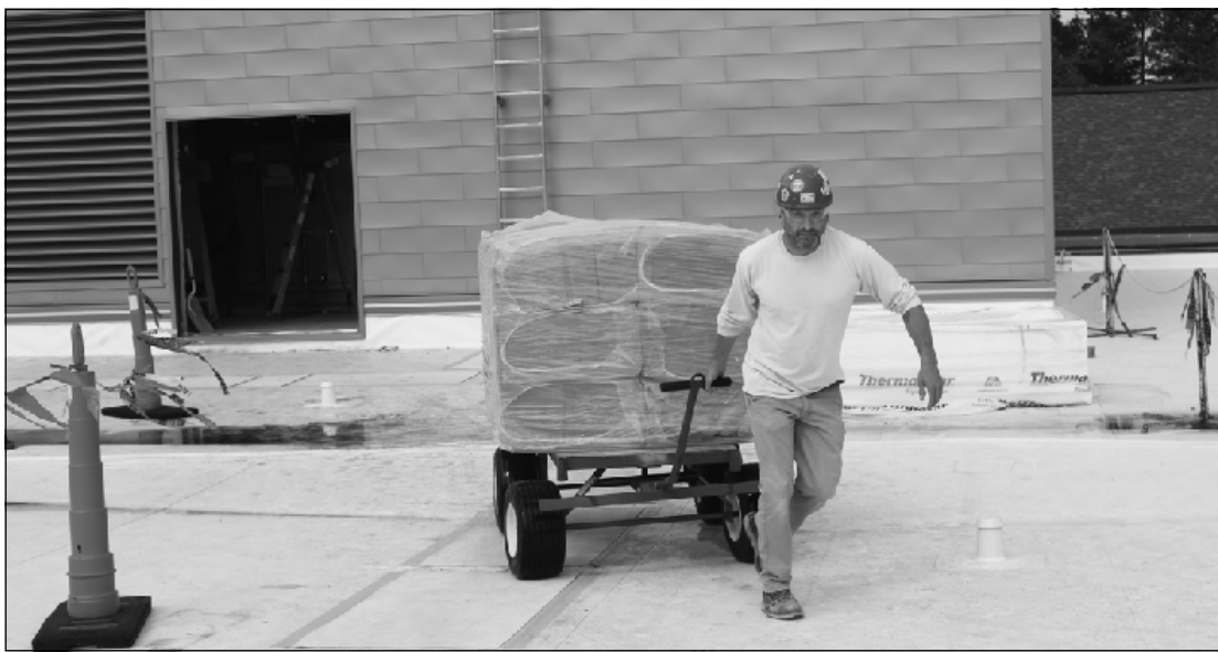
SPECIAL DELIVERY – David Frick of Heat and Frost Insulators Local 47 moves a lot of insulation board the easy way, working on the roof of a building at the Caro Psychiatric Hospital. He's employed by Mechanical Insulation.
