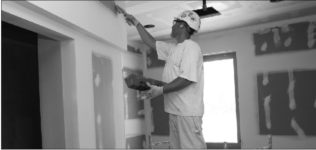
MUDDING A DRYWALL joint in a patient room at the Caro Psychiatric Hospital project is Harold Loney of Michigan Painters District Council Local 2353. He's employed by Commercial Contracting Corp.
