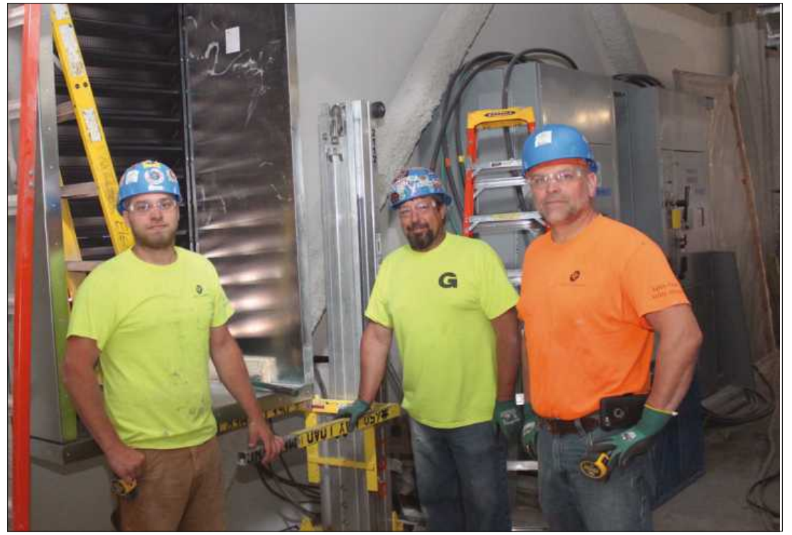
WE ASKED THIS GROUP of Sheet Metal Workers Local 7 members to pause what they were doing for a photo in front of some of their handiwork – a large insulated plenum they installed at the Caro Psychiatric Hospital. They are (l-r) Colby Hemgesberg, Dave Moening and Kevin Scharich. They're working for Dee Cramer.
