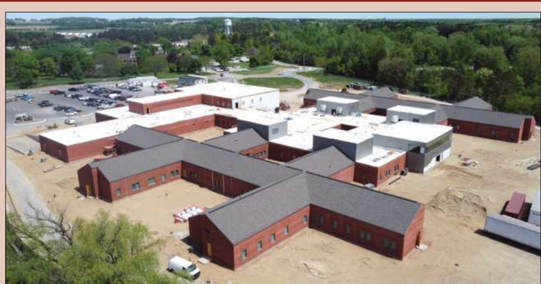
A NEW 127,000-square-foot, 100-bed Caro Psychiatric Hospital is under construction, progressing under the management of Granger Construction. The new facility replaces an older facility nearby. Photo credit: Granger Construction
