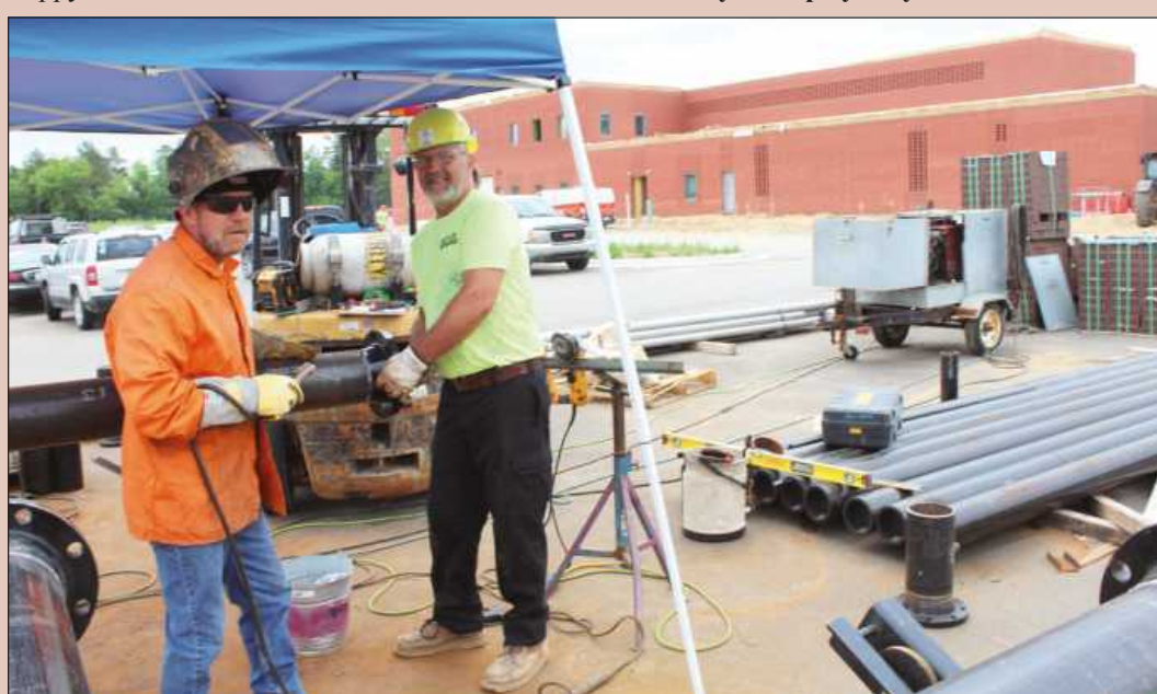
READYING A WELD on a 6-inch chilled water pipe at the Caro Psychiatric Hospital project are (l-r) Brant Scheurs and Rob Crummel of Plumbers and Steamfitters Local 85. They're employed by Remer Plumbing and Heating. We will have more project photos in our next edition.
