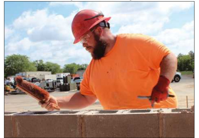
GIVING THE BRUSH to a wall that will contain dumpsters at the new Caro Psychiatric Hospital is Ray Robison of Bricklayers & Allied Craftworkers Local 2. He's employed by Boettcher Masonry.
