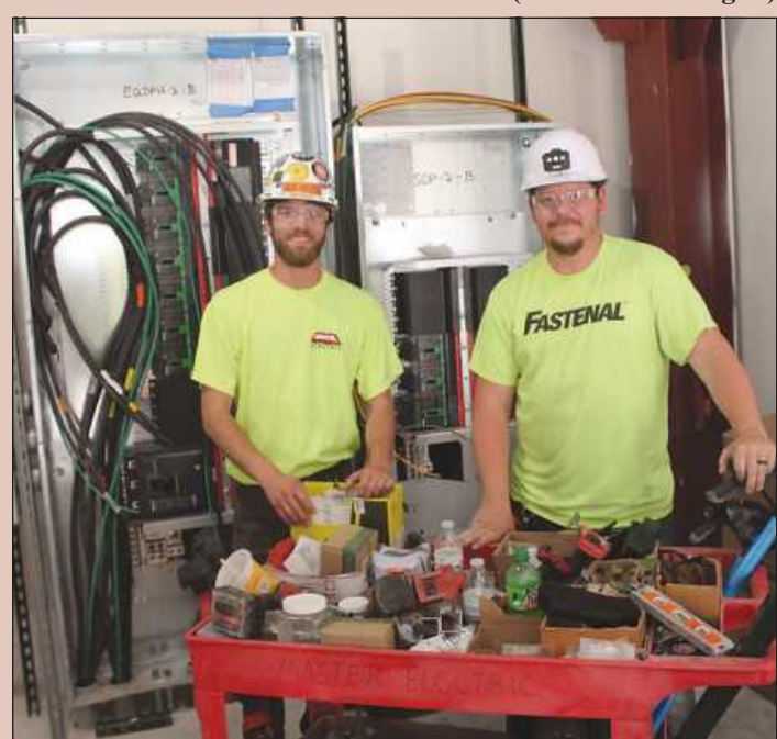
IN FRONT OF THE switchgear panels that they helped install at the Caro Psychiatric Hospital project are (l-r) Reed White and Nick Iles of IBEW Local 557. They're employed by Master Electric.
