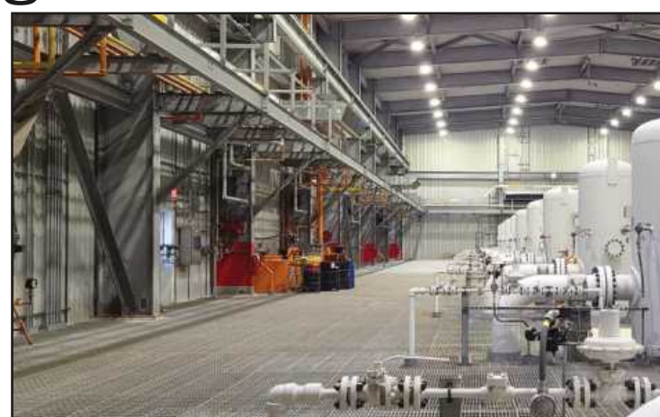
NEWLY INSTALLED equipment at the Freedom Compressor Station. Photo credit: Consumers Energy
