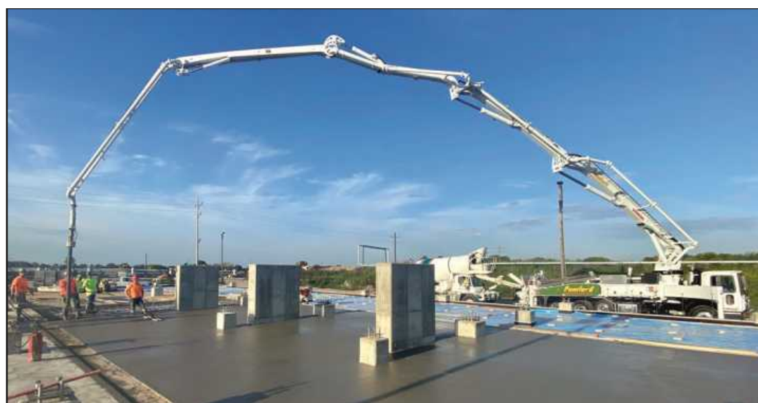
CONCRETE IS PUMPED into place at the Michigan Sugar de-sugarization project in Bay City during foundation work last month. Doing the work are Bricklayers and Allied Craftworkers Local 2 masons and Laborers Local 1098 members.
