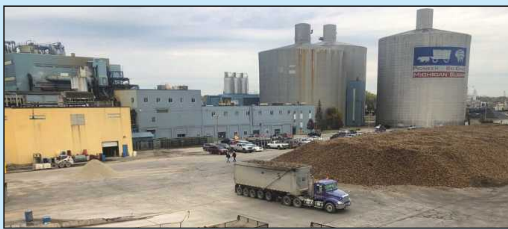
MICHIGAN SUGAR CO., whose products Pioneer and Big Chief, is expanding its Bay City Plant with a new $75 million "desugarization" facility. The company makes sugar from processing sugarbeets harvested from area farms. The plant under construction will allow the company to extract more sugar from one of their byproducts, molasses.
