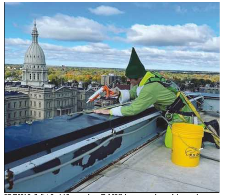
IBEW LOCAL 665 member Ed White goes about his work as an electrician and Santa's helper while getting the city ready for its annual Silver Bells in the City celebration. Here he sets a string of lights atop a building across from the Michigan Capitol Building.
