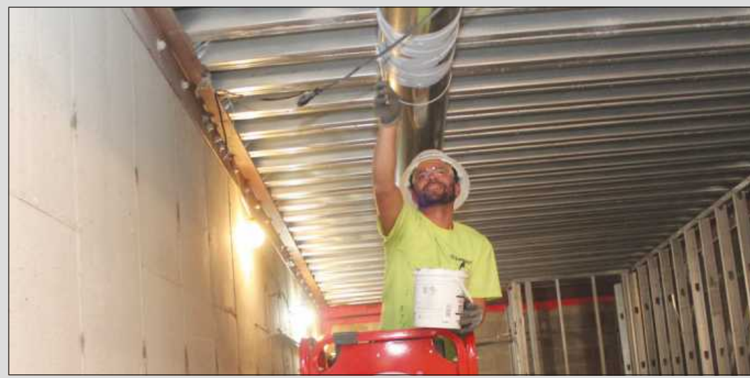
SEALING A DUCT in a service connector stairwell at the Heritage Hall project at the Michigan Capitol Building in Lansing is Chris Rosado of Sheet Metal Workers Local 7. He's employed by Limbach.
