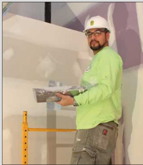
MUDDING WALL at the Heritage Hall project in Lansing is Rolando Gonzales of Michigan Painters District Council Local 845. He's employed by Integrity Interiors.
