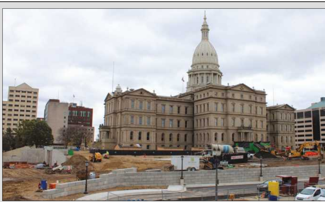
MOSTLY BELOW THE WEST SIDE of the grounds of the Michigan Capitol Building in Lansing, the Christman Co., their subcontractors and building trades union workers are building Heritage Hall, which will have meeting space but act primarily as a starting-off point for visitors and school tours at the 1879 building.
