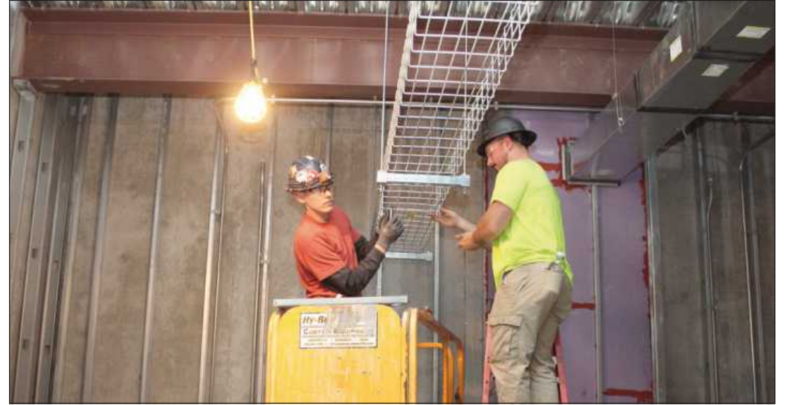
SETTING UP CABLE TRAY at the Michigan Capitol Heritage Project in Lansing are Dalton Bailey and Cody Savage of IBEW Local 665. They’re employed by Summit Electric.
