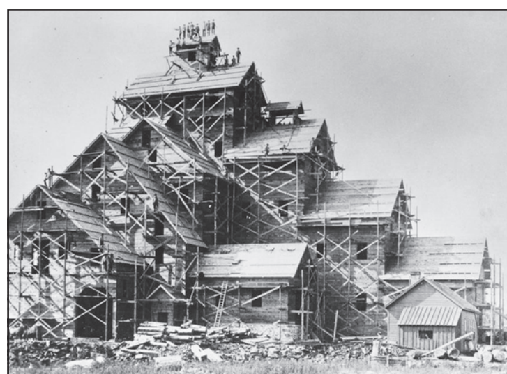
THE ELABORATELY scaffolded Quincy Mine Rockhouse No. 6 was a trendsetter in the copper ore industry. Shown here under construction in 1892, it was later demolished.
