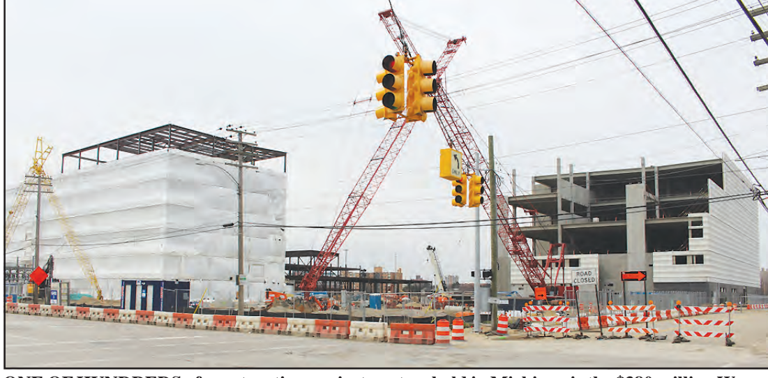
ONE OF HUNDREDS of construction projects put on hold in Michigan is the $380 million Wayne County Criminal Justice Complex at I-75 and East Warren. Managed by Barton Malow, the project had been slated for completion in mid-2022. The project includes an adult detention facility, office space and a courthouse.
