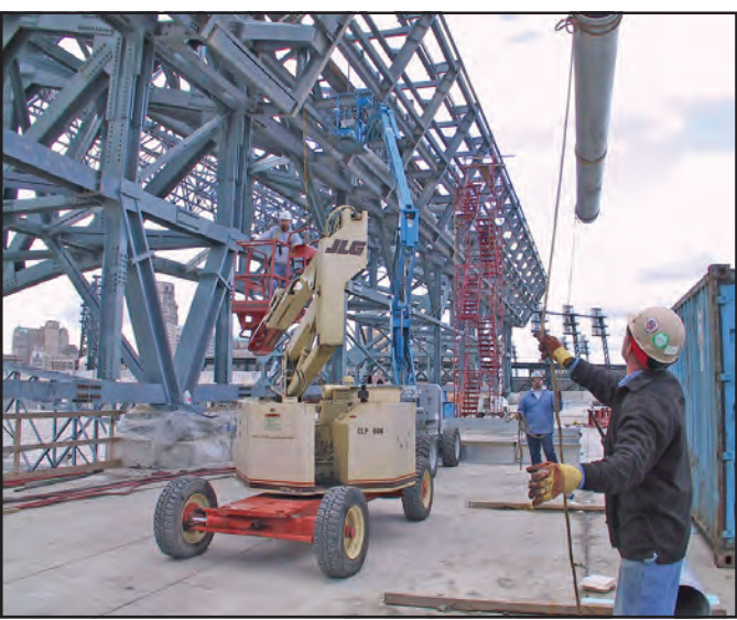
PLUMBERS 98 workers swing pipe in what will be the Comerica Park concourse.
