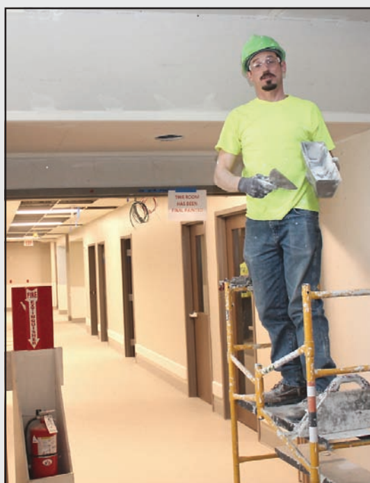
MUDDING SEAMS ON ceiling in a second floor lobby of the Promedica Hospital project in Adrian is Bryan Stone of Michigan Painters and Allied Trades IM-Local 514. He works for OCM Contractors.
