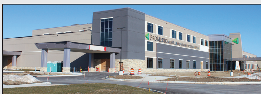
THE NEW PROMEDICA Charles and Virginia Hickman Hospital is being erected on a former golf course in Adrian Twp. Managed by Lothrop, the project is expected to be complete in early June.
