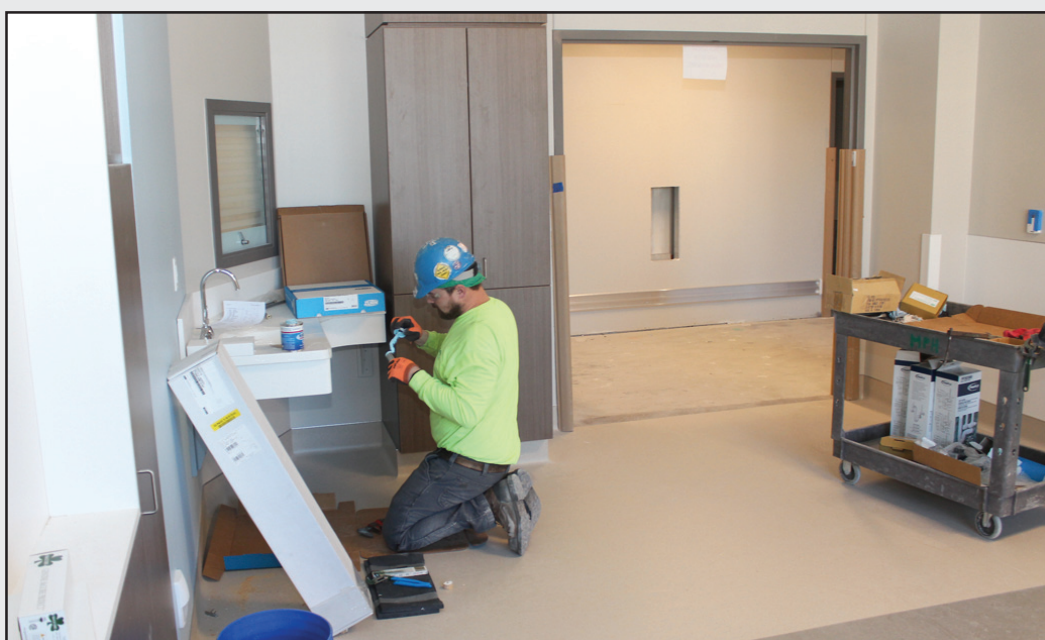
TRIMMING OUT a sink faucet on the third floor of the new Promedica Hospital in Adrian is Jake Jondro of Plumber and Pipe Fitters Local 671. He's employed by Monroe Plumbing and Heating. The photos were taken prior to the onset of the COVID-19 quarantine.
