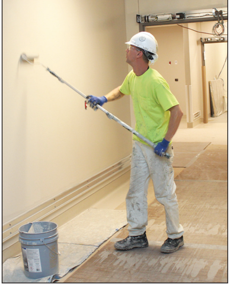
PAINTING A SECOND FLOOR hallway wall at the Promedica Hospital project in Adrian is Jason Tivis of Painters and Allied Trades 1-M, Local 514. He's employed by Bucher.
