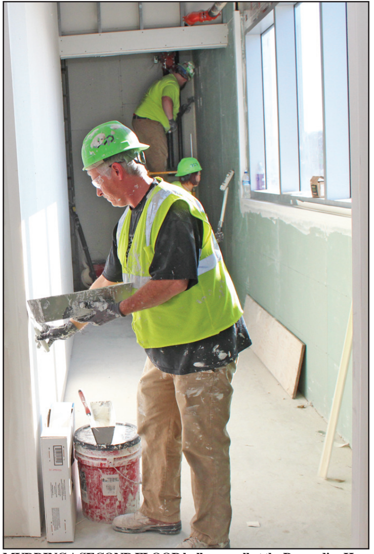
MUDDING A SECOND FLOOR hallway wall at the Promedica Hospital project in Adrian is Bill Roberts of Painters and Allied Trades 1-M, Local 514. He's employed by OCP Contractors.
